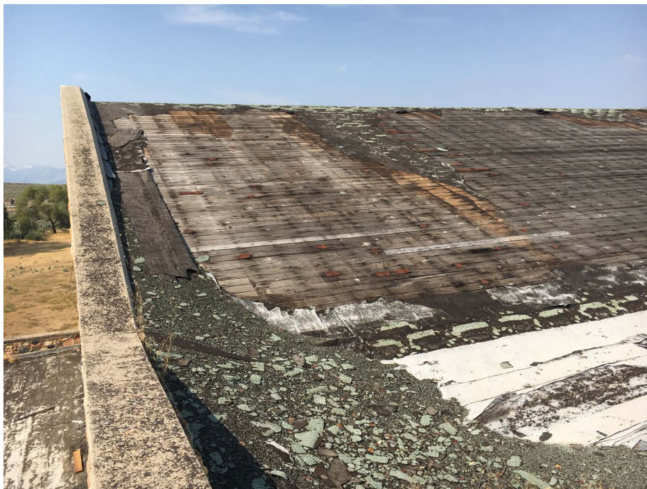
Elevation: Roof and lower parapet Detail of Old Gym roof condition prior to roof replacement project Photographer: Kirsten E. Nalley, SPWD Date: 8/3/2017
