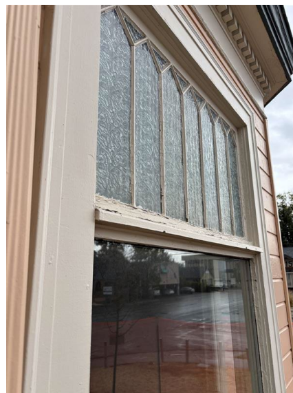
Figure 8: Special window in first-floor bay with textured glass upper sash. Photo credit: Melissa Hafey 10/02/2025.
