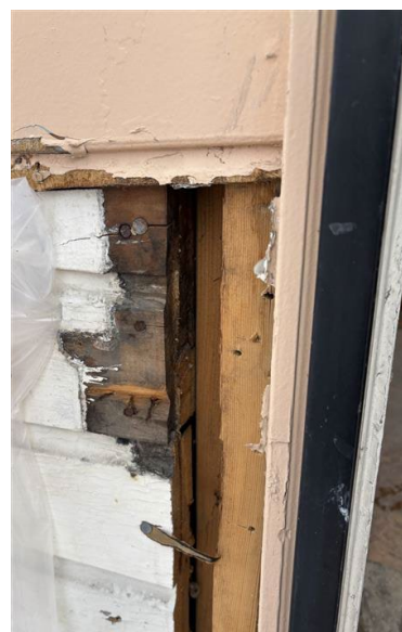
Figure 7: Original shiplap cladding under a newer layer of siding. Photo credit: Melissa Hafey 10/02/2025.
