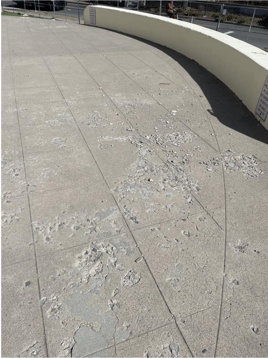
Main landing at south facade entrance, showing concrete damage and previous repair.
