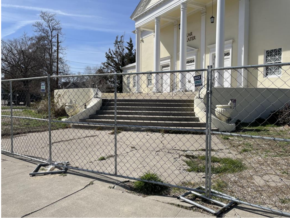
Front (south) facade, right sidewalk and stairs up to main entrance. Shows damaged concrete.
