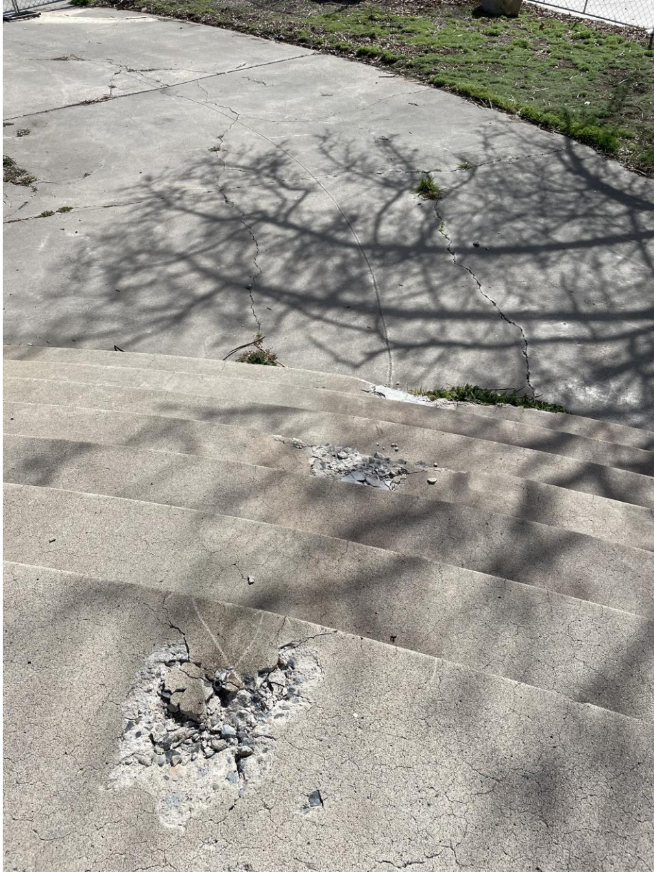
Detail of western stairs and sidewalk off of main landing on south facade.
