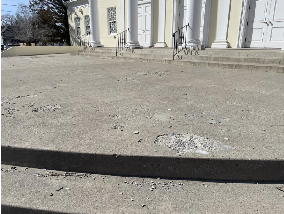
South facade main landing, showing concrete damage.
