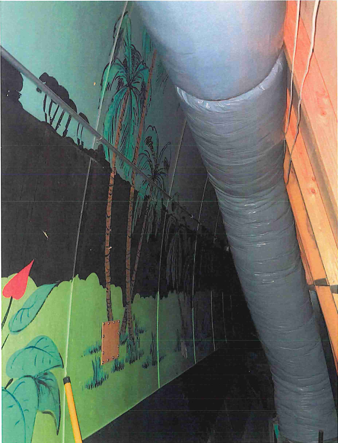
Original curved exterior wall with 1962 mural, with 1960s interior framed wall on right Kansas Bowling, 2023
