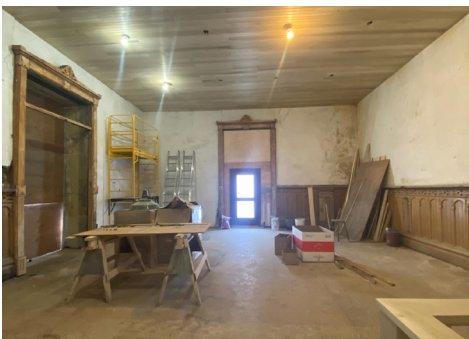
The rear room, complete with its original wood wainscoting and huge wood and glass French doors, is being rehabilitated with CCCHP grant funds to provide space for a dance and art studio.
