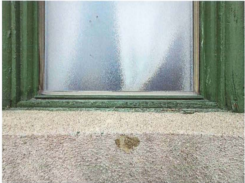
Weathered and Cracking Trim
