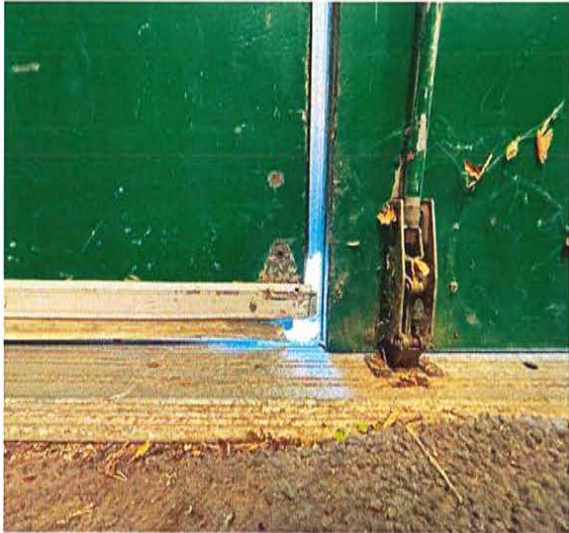
Brewery Annex Double Doors warped/bent gaps
