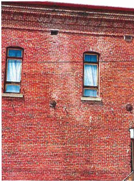
Missing Downspout connection
