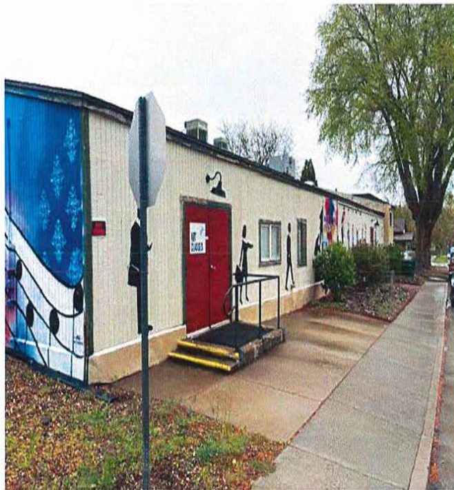
Hole in Gutter at Pottery
