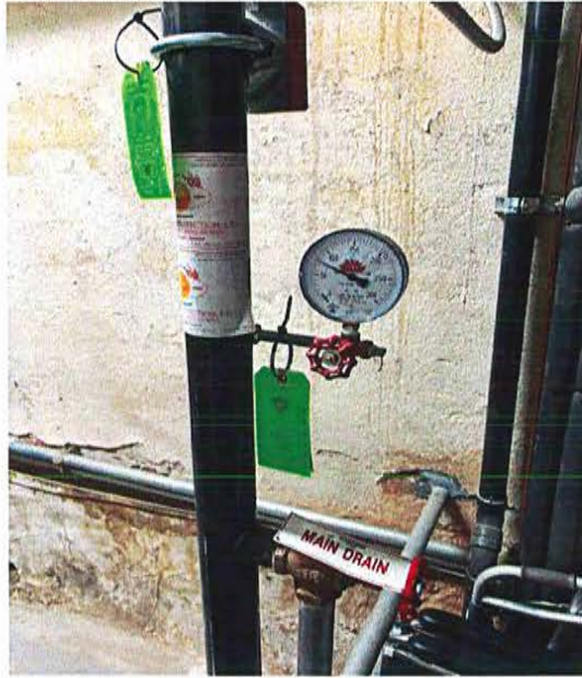
Brewery Building Fire Sprinkler Valve
