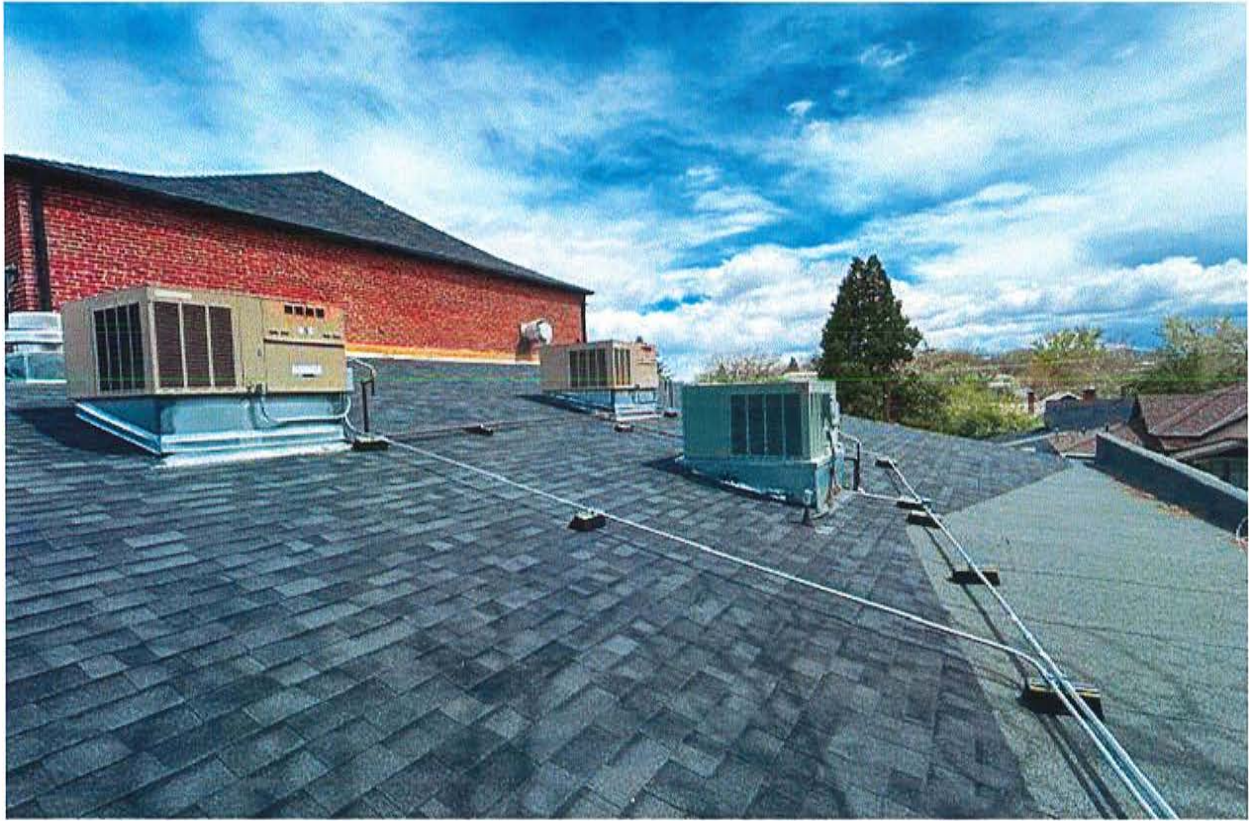
3 Package Units on roof of Black Box Theater – One is dead, the other 2 are dying all 3 are same age
