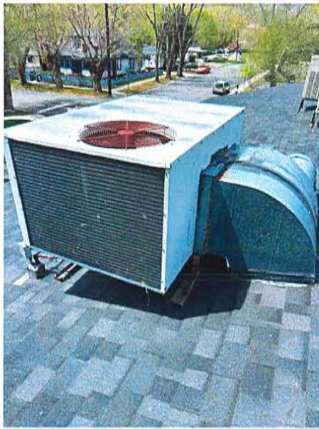
Rooftop Unit NAA Gallery looking west
