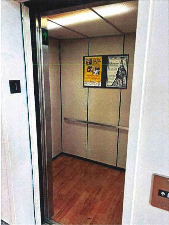
Building Elevator Car Elevator In-Car Controls
