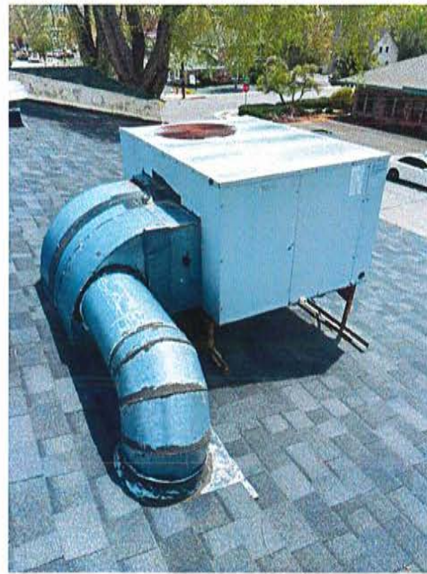
Rooftop Unit NAA Gallery looking South
