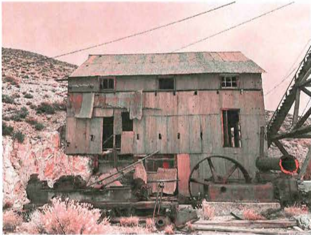
Hoist House facing southeast showing exterior damage
