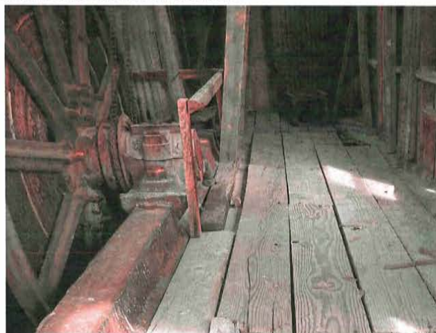
Interior of Hoist House showing damaged floorboards
