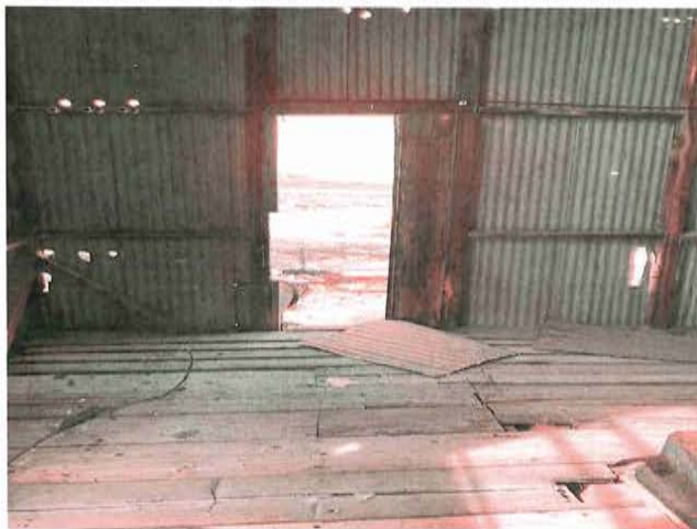
Hoist House interior facing southwest showing flooring and siding damage
