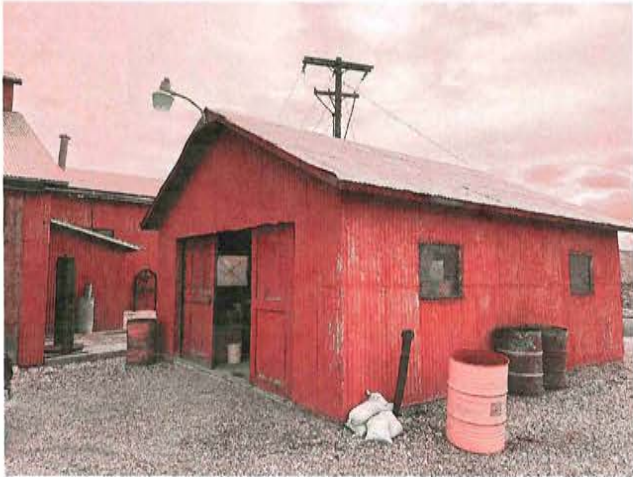
Service Bay facing southeast showing window and sliding door damage
