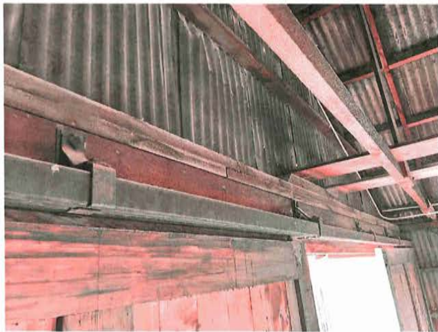
Service Bay interior facing east showing interior of sliding door and potential area to install viewing panel
