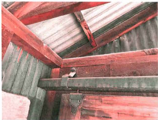
Service Bay interior facing northwest showing interior of sliding door and potential area to install viewing panel
