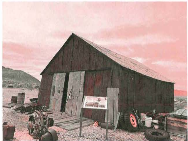
Rope Shed facing northwest showing slanting and instability
