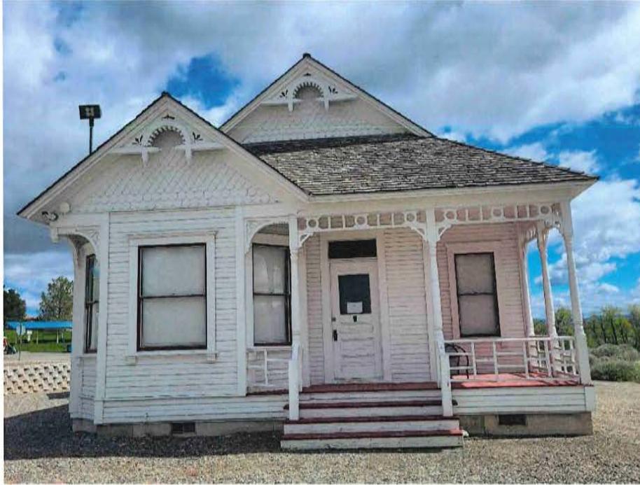
Richardson House roof in need of preservation oil treatment-
