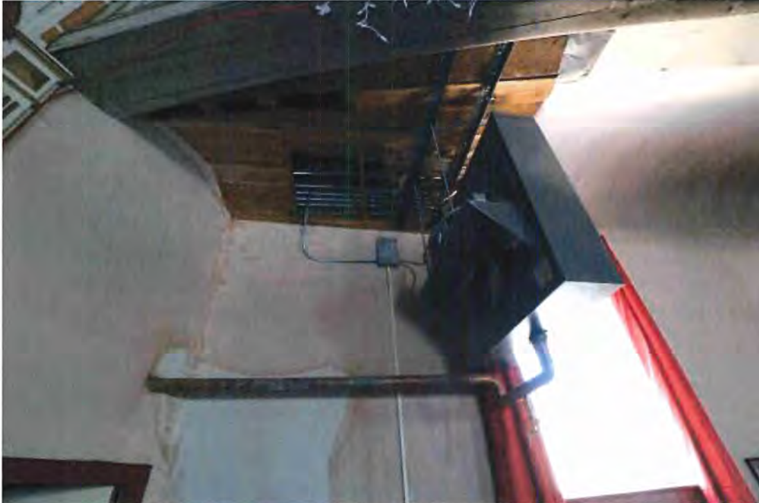
Photo 50 View of exposed lath under balcony at north side above door to stage and boxes. Unit heater visible to right in photo.
