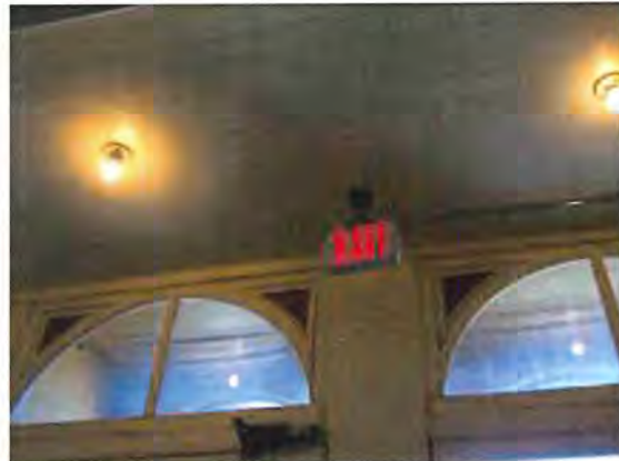
Photo 12 No emergency light at Main Entrance
