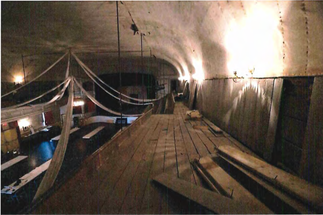
Photo 64 View of north balcony looking west toward doorway which exits behind upper opera box. Boards should be reattached to wainscot and missing pieces custom milled.
