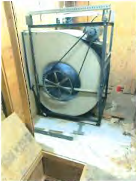
Photo 6 Exhaust Fan in Attic
