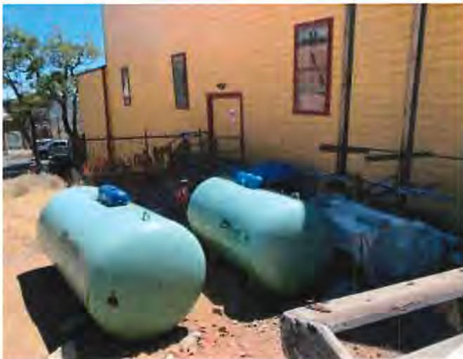
Photo 1 Propane Storage Tanks on north side of Piper's Opera House
