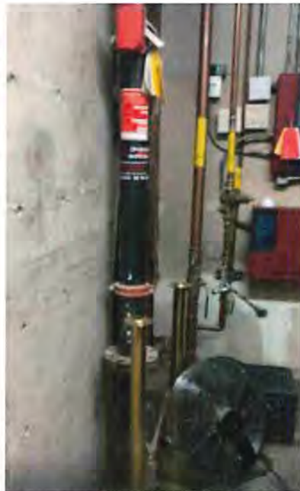
Photo 3 Fire Riser and Domestic Water Riser
