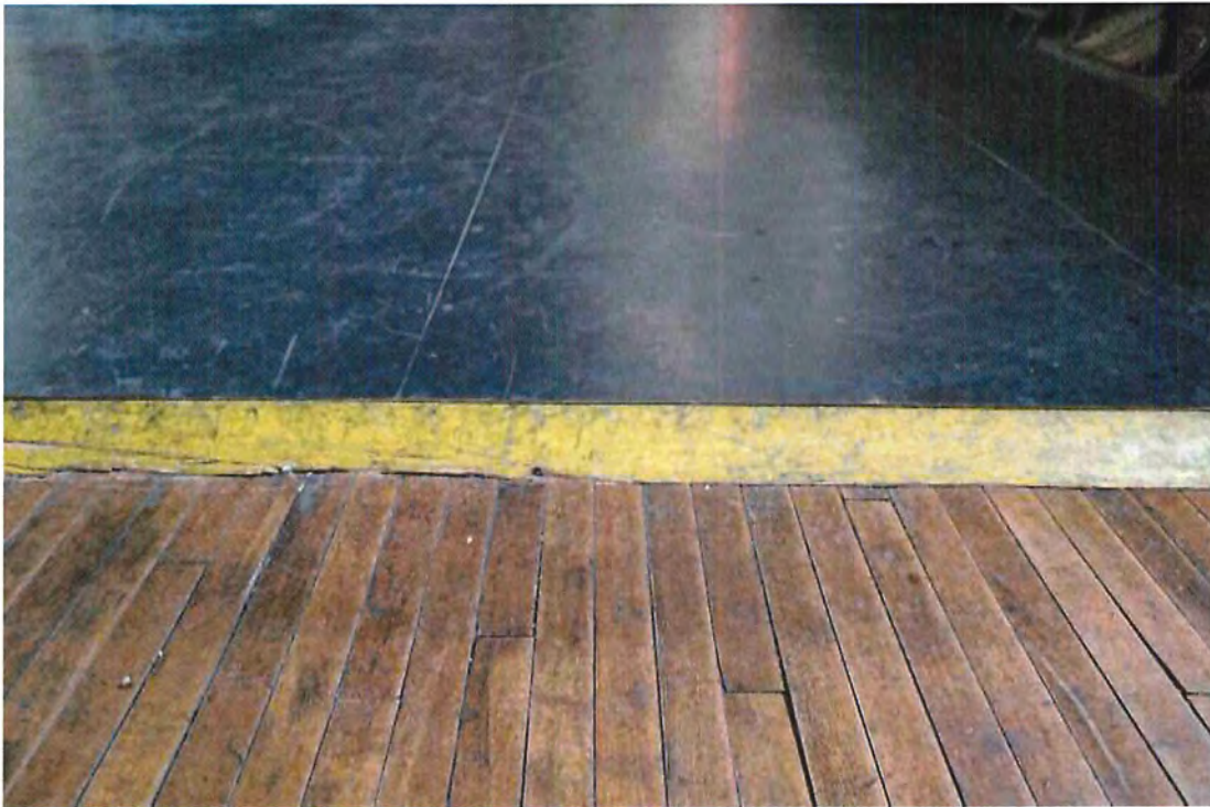
Photo 48 1907 maple flooring visible in foreground. In 2007, HBO set up production studio and added 2 layers of plywood, painted black, over maple flooring. Note beveled transition strip painted yellow. Maple flooring appears to be in fair to good condition.
