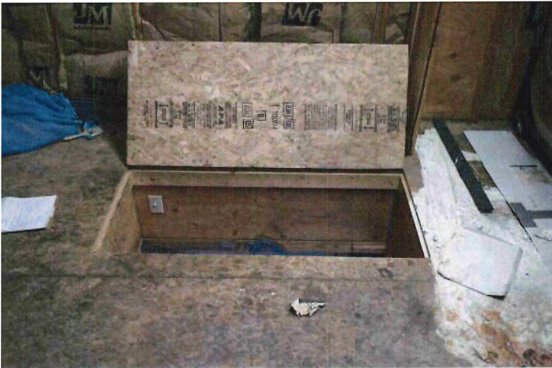
Photo 67 View of ladder access from platform in attic. Note location of light switch
