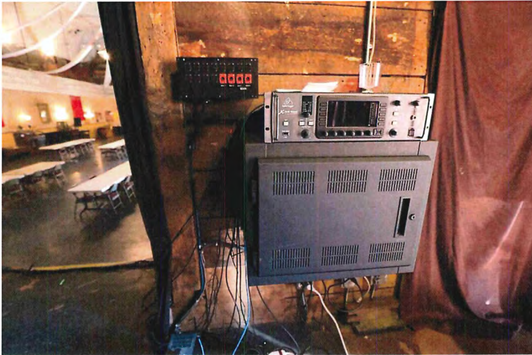
Photo 56 40-channel digital live mixer rack installed stage right
