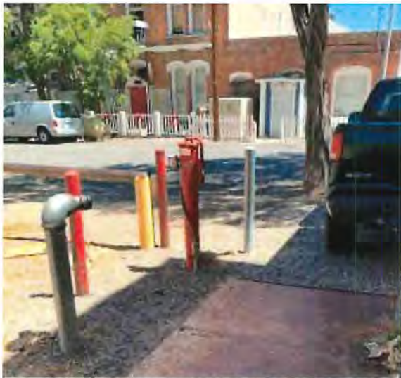
Photo 2 Fire Department Connection and Post Indicator
