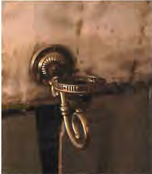
Photo 63 balcony light fixture missing glass shade and bulb
