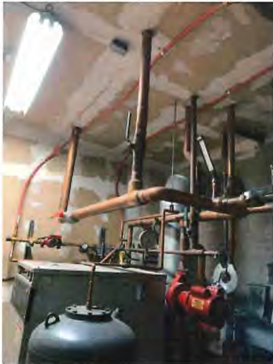
Photo 4 Boiler and Hydronic Equipment
