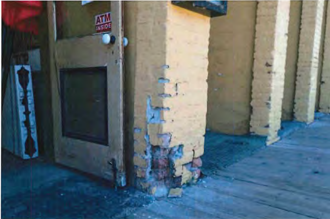
Photo 24 Damaged brick column on B Street façade at entry to Old Corner Saloon
