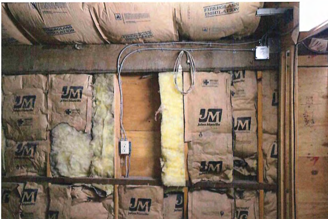
Photo 68 Kraft-faced fiberglass batt insulation at walls (R19) and roof (R38). Note plywood sheathing
