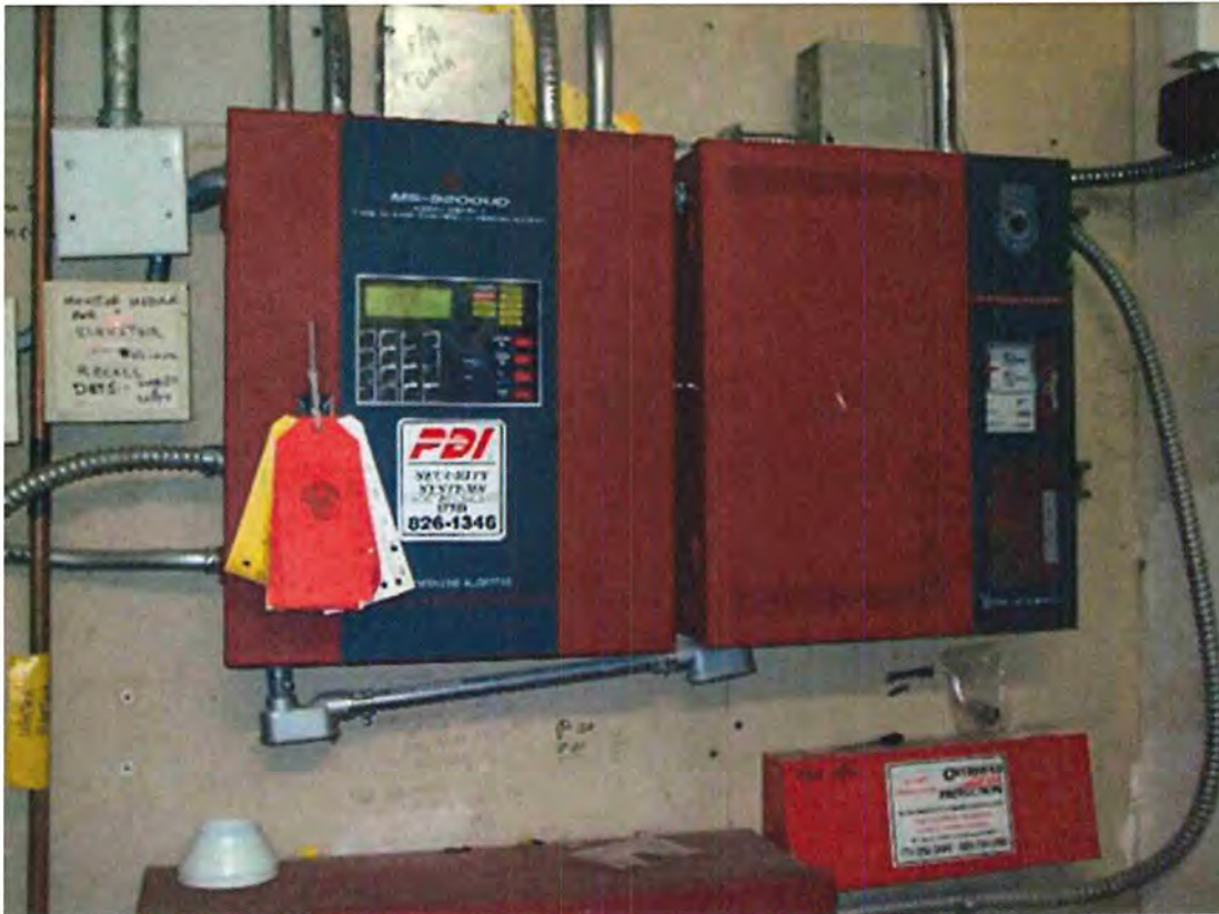
Photo 17 Existing Fire Alarm panel in Fire Riser Room
