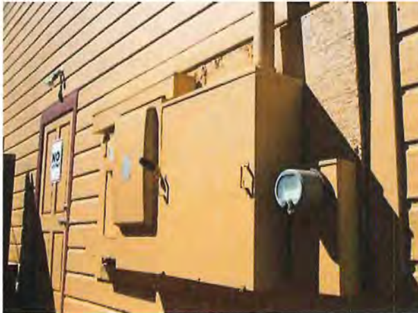
Photo 8 Existing 120/208 volts, 3 phase, 4 wire, 400 amp electrical service on south auditorium elevation
