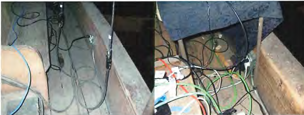
Photo 10 Extension cords and cables lying about in the balcony
