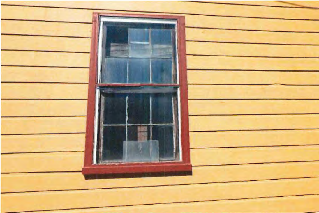
Photo 32 Exterior mounted 1 over 1 storm window, typical of three on south side and three on north side. Note deteriorating condition of window sashes beyond.
