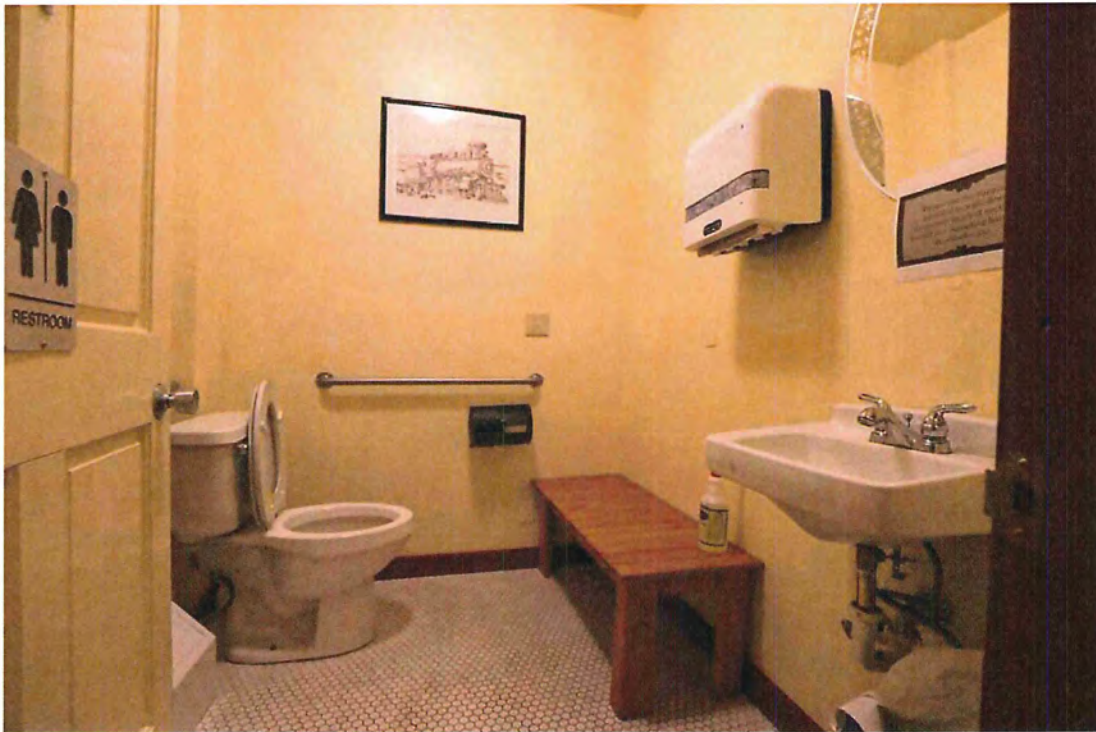
Photo 44 Auditorium level single occupancy restroom. Does not meet accessibility standards
