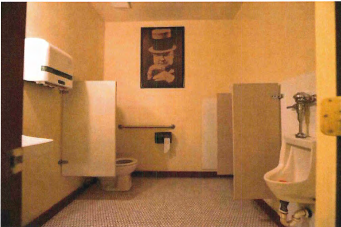
Photo 45 Auditorium level Men's Restroom. One lavatory, three urinals, and one water closet. As configured, single occupancy restroom while water closet in use. Does not meet accessibility standards as currently configured. Door is too narrow into restroom.
