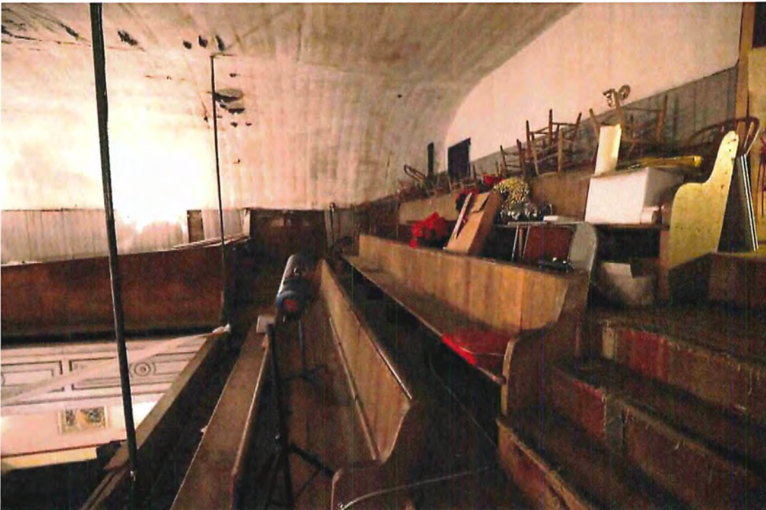
Photo 65 Stairs descend from main balcony entrance to right in photo. Pew bottom missing. Note damaged guardrail cap left of rod supporting balcony
