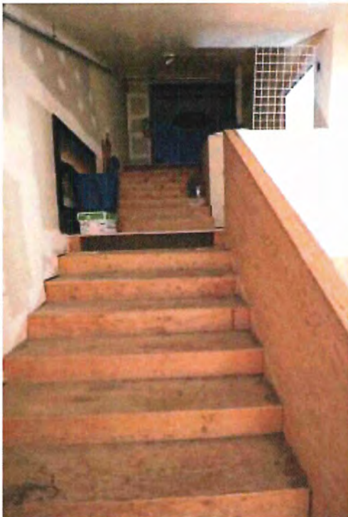
Photo 62 Unfinished stairs to balcony level. Door to current VCTC office shown at right on intermediate landing
