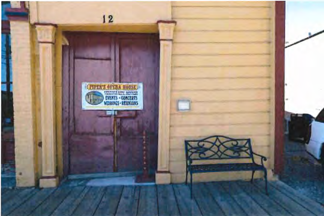
Photo 31 Carriage House doors. Note the cast iron piers. Doors are in poor condition and arch obscured by plywood panel
