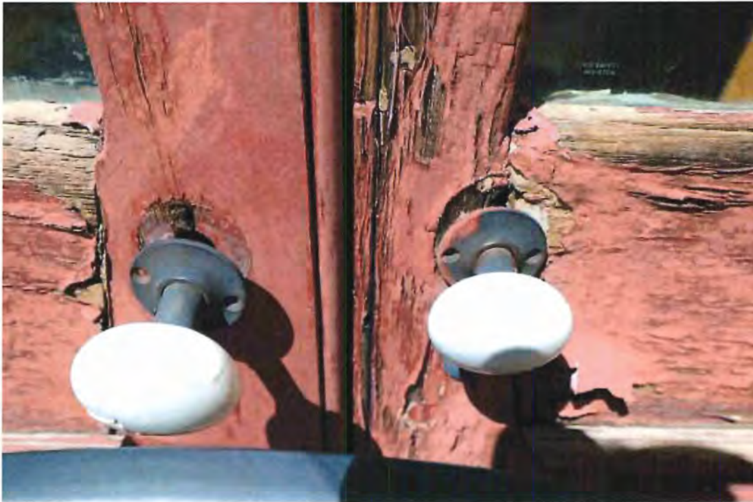
Photo 30 Main entry doors at B Street. Screws missing at door knob escutcheons. Paint peeling.
