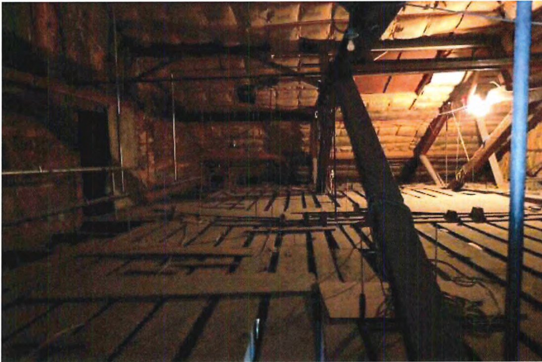
Photo 69 View of loft area above stage taken from ladder platform looking south.
