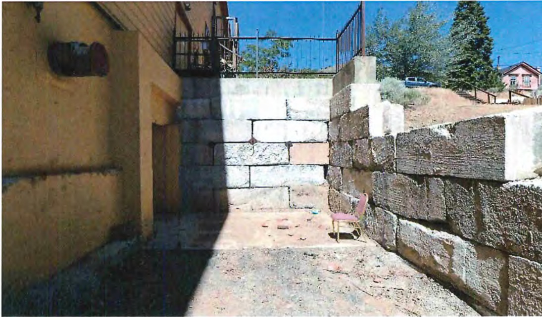
Photo 37 Excavation at north side for access to double egress doors. Existing concrete pad with snow melt system. Pour new 3 inches of a/c pavement over 6 inches of compacted aggregate base from edge of concrete pad to B Street
