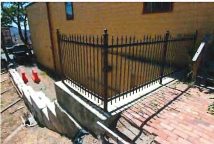
Photo 27 Note missing finials
