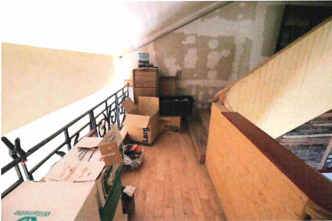
Photo 61 View of landing to balcony level. Note clamp at guardrail.
