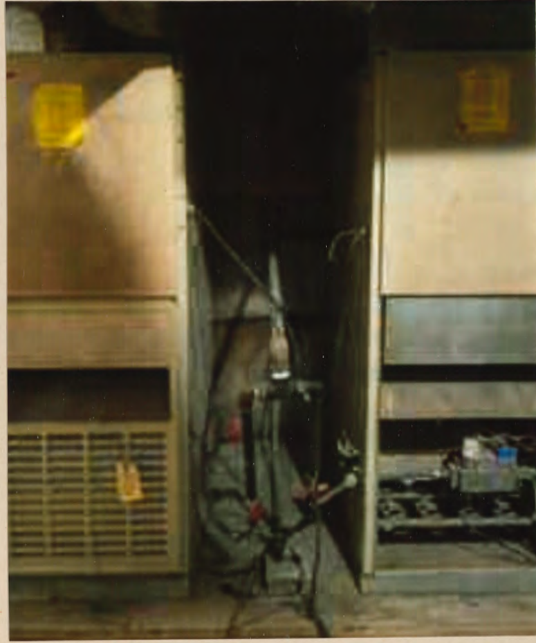
Top two pictures are of downstairs theatre cooling system, probably installed in 1940's. Unit is badly rusted thru out & needs replacement. We have been told it would be very hard & expensive (if even possible) to repair this unit. Picture to left is of furnace unit for lower theatre (one on right does not work). Furnace functions but is older and has problems.
