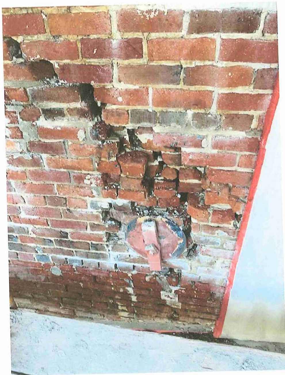
Blown-out large crack in brick wall
