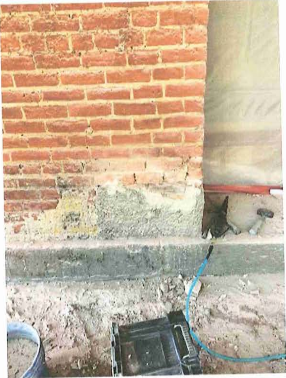
Bad concrete patch on corner
