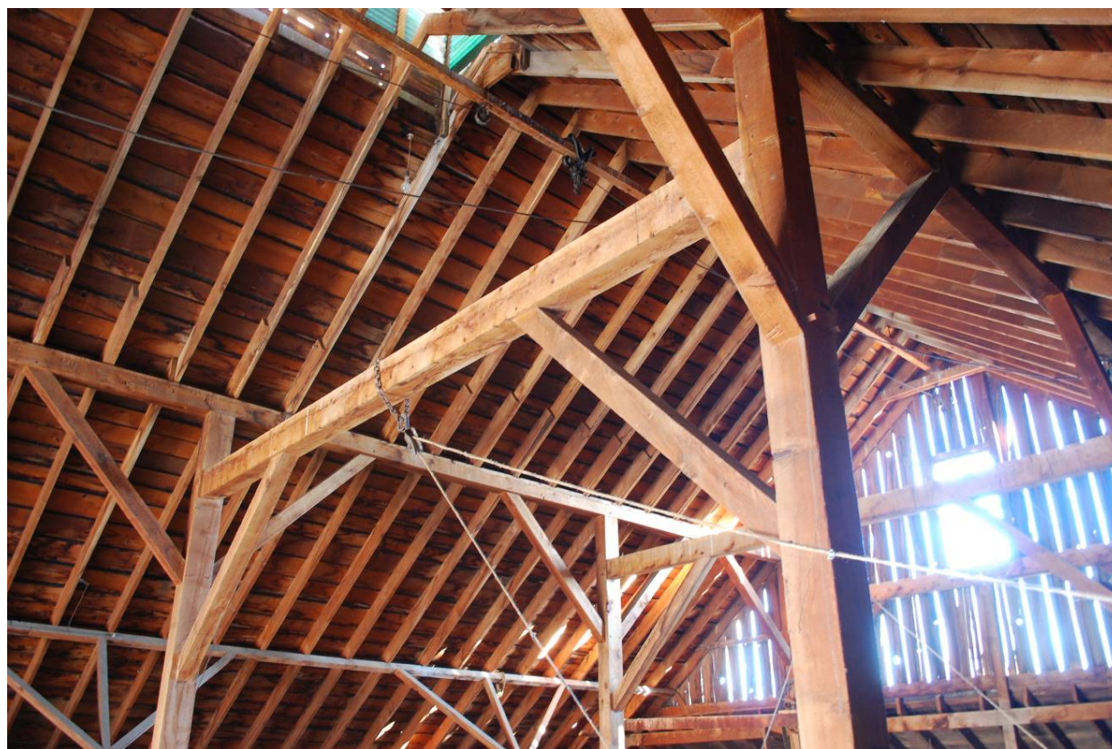
Photograph 6 – Barn interior, viewing primary framing and roofing structure, looking up and southeast.
