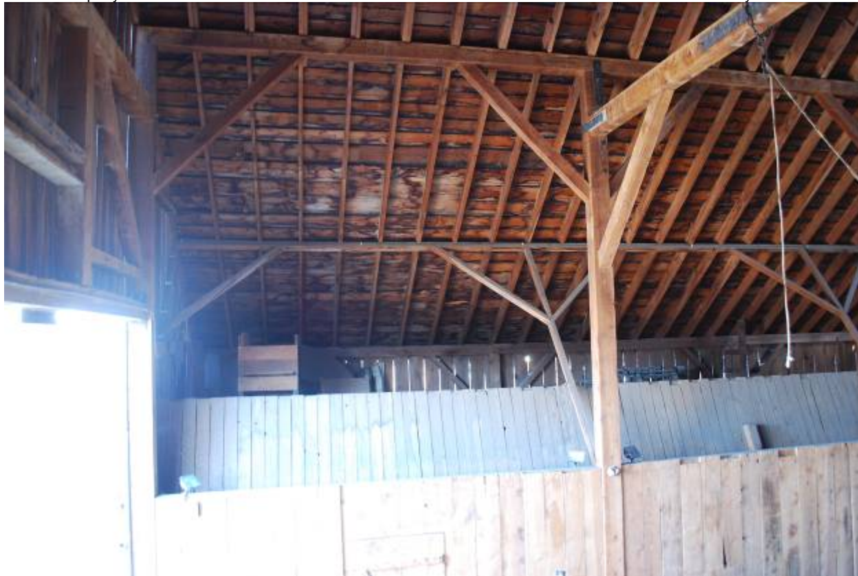
Photograph 27 – Barn roof framing system, showing dropped tie beam (upper right and left) and unique angled truss bracing system along secondary (lower) purlin.
