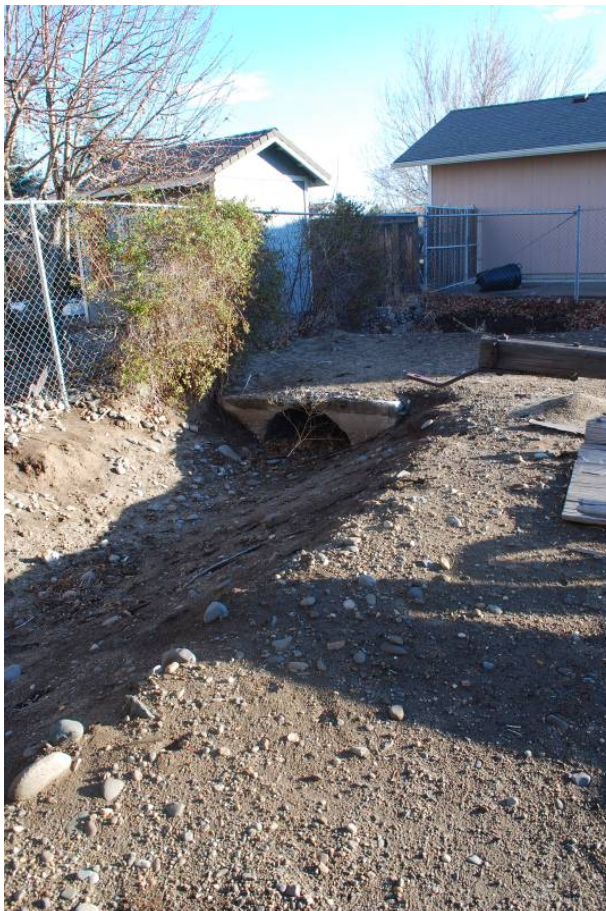
Photograph 21 (right) – Remnant of the Hussman Company Ditch and a concrete culvert and bridge at southeast edge of property. Formerly, the road leading from the main house and barn led across this bridge and into alfalfa fields to the east.
